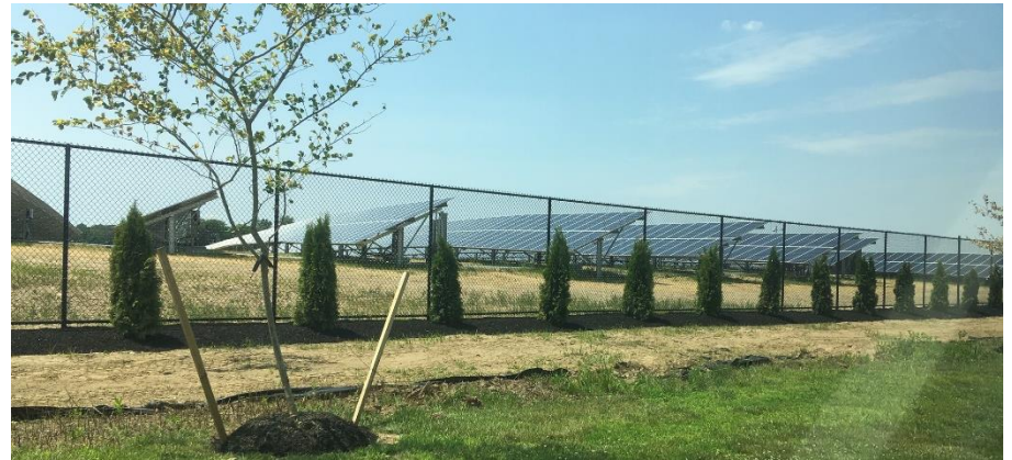
AC Power's 4.75 MWdc solar project in Delanco Township
